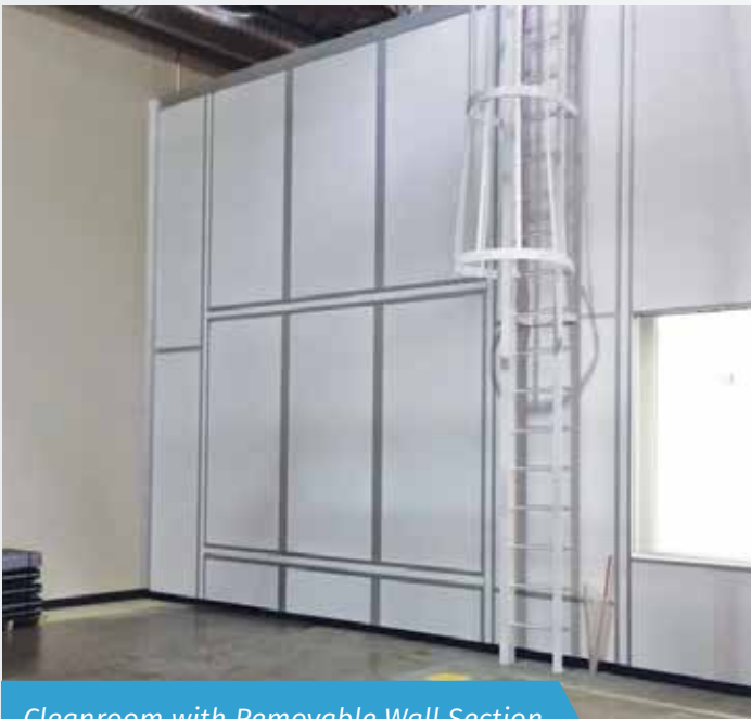
Cleanroom with Removable Wall Section
