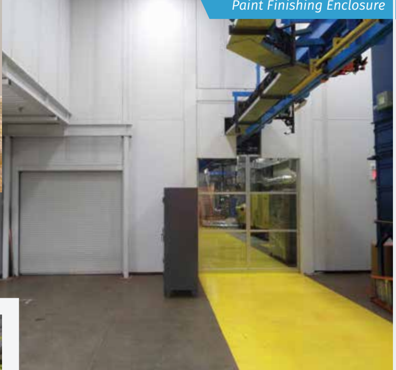
Environmentally Controlled Paint Finishing Enclosure
